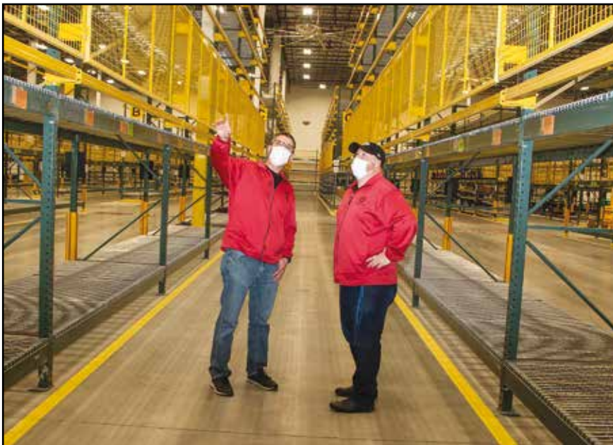
Local 249 Bargaining Chair Jim Fisher, left, and President Jason Starr inspect progress on a new sequencing facility for the E-Transit being constructed on Highway 291. Photo by Don Lehman.
