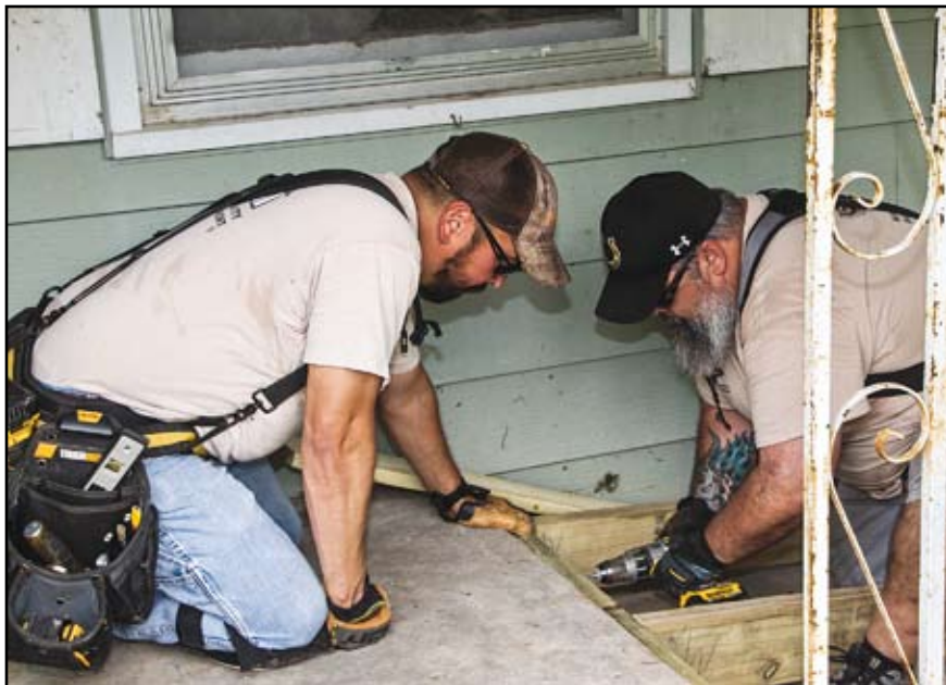
Phil Rangel, left, and Jeff Chisam, members of Local 249's Ramp Crew work on the deck of a ramp. The crew has built hundreds of ramps for housebound individuals in the area. Photo by Don Lehman.
